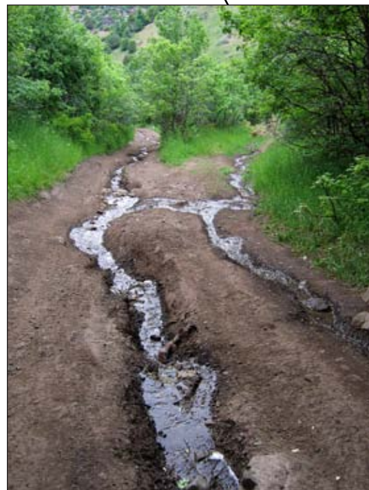
Poor drainage and braiding routes created
