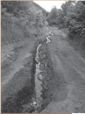
Above: Ruts from OHV abuse create widened roadways damaging vegetation and create maintenance nightmares.
