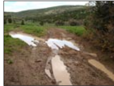
R-4 Poor drainage
